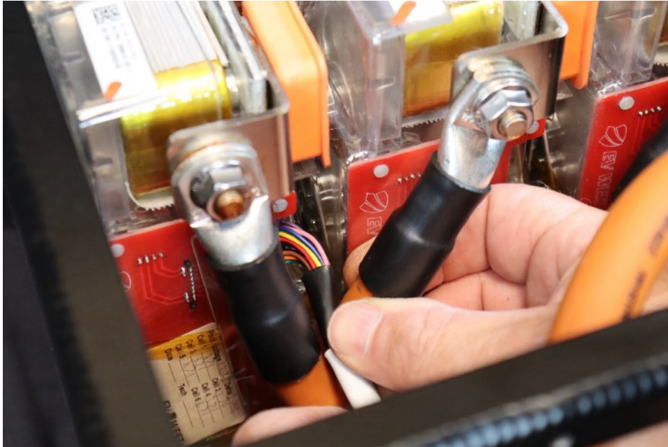
Plug in front battery BMS.
