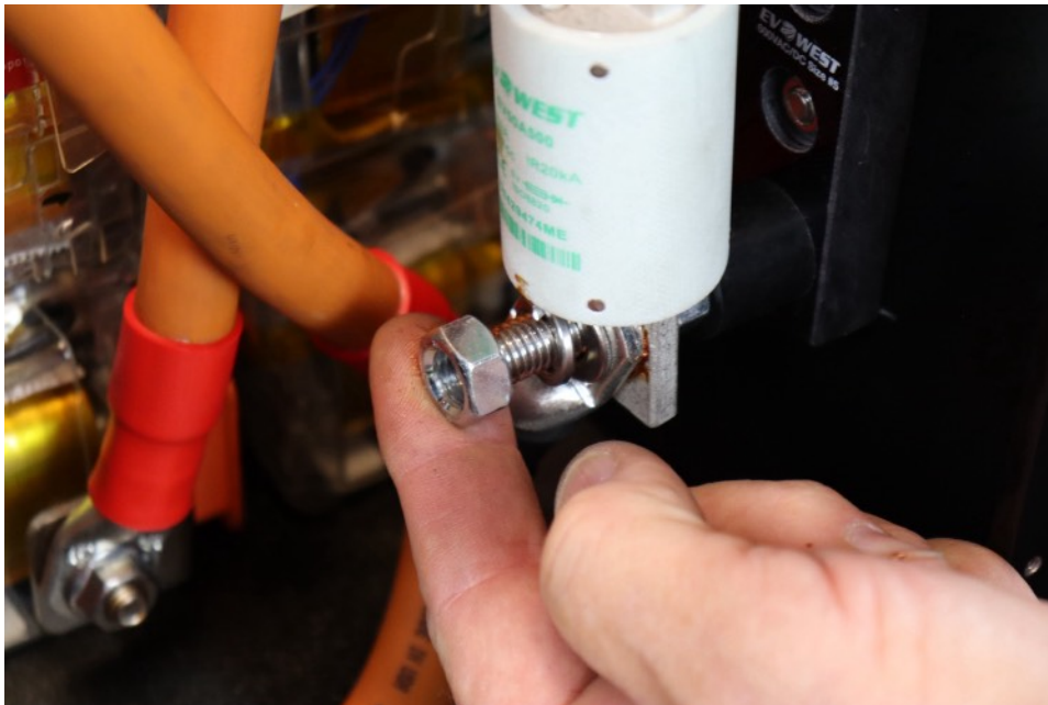
Install Amphenol Negative cable to the fuse holder.
