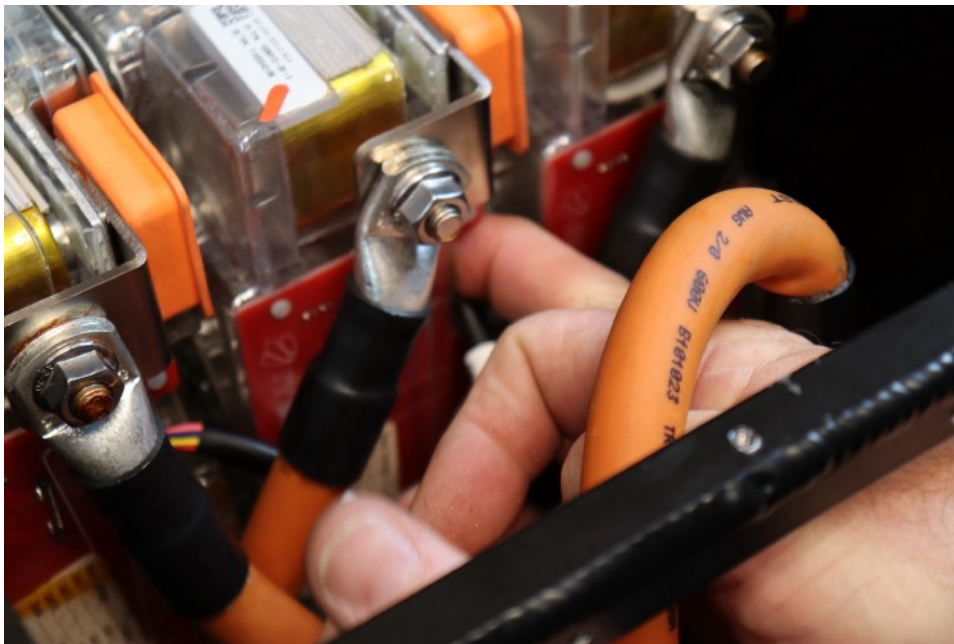
Plug in middle battery BMS.
