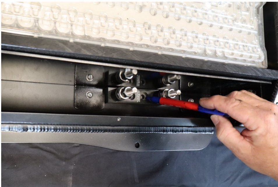
Mark and drill fuse holder mount holes. Leave clearance between fuse holder and BMS mount for fuse body
